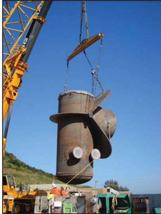
A 33-ton, vertical riser pipe has been secured inside the tunnel at the West Shaft to connect the pipeline with the Water Authority's aqueduct system.
