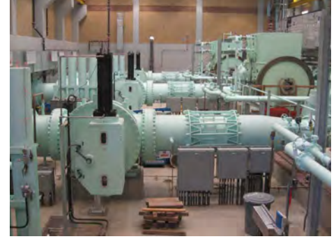
The pump station will help move water from San Vicente Reservoir in an emergency.
