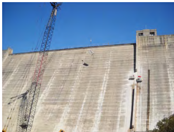
Crews remove concrete sections of the dam to prepare for the raise.
