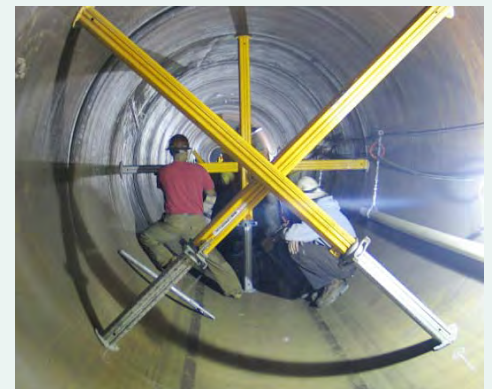
To protect the pipe during grout work, eight-foot-tall aluminum beams are placed in a crossed position inside the pipe.
