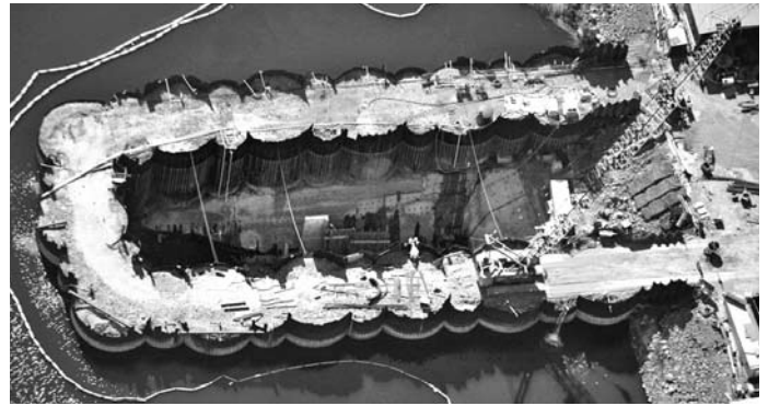
The temporary cofferdam in the reservoir will be removed this spring. It kept water out of the area that was used to build the inlet-outlet structure on the bottom of the lake.
