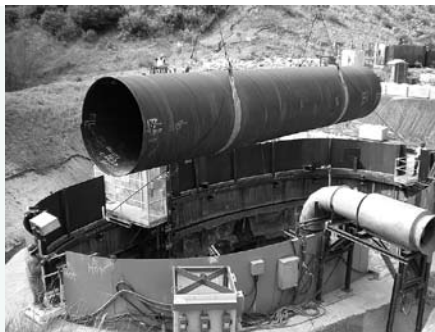
Pipe segments are lowered into the Central Shaft and transported as far as five miles through the tunnel.
