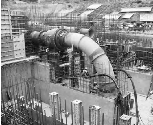
The 48-inch diameter pipe inside the pump station connects to one of the two 28,000 horsepower pump turbines.
