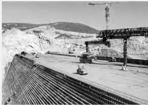
Roller-compacted concrete was used to build Olivenhain Dam and will be used again to raise San Vicente Dam.
