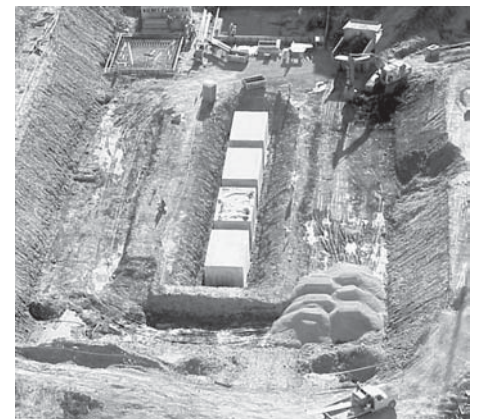
Site view of pump pads at the Olivenhain Pump Station.
