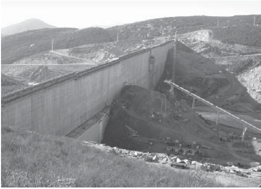
The entire upstream side of the dam will be covered with the Carpi liner.
